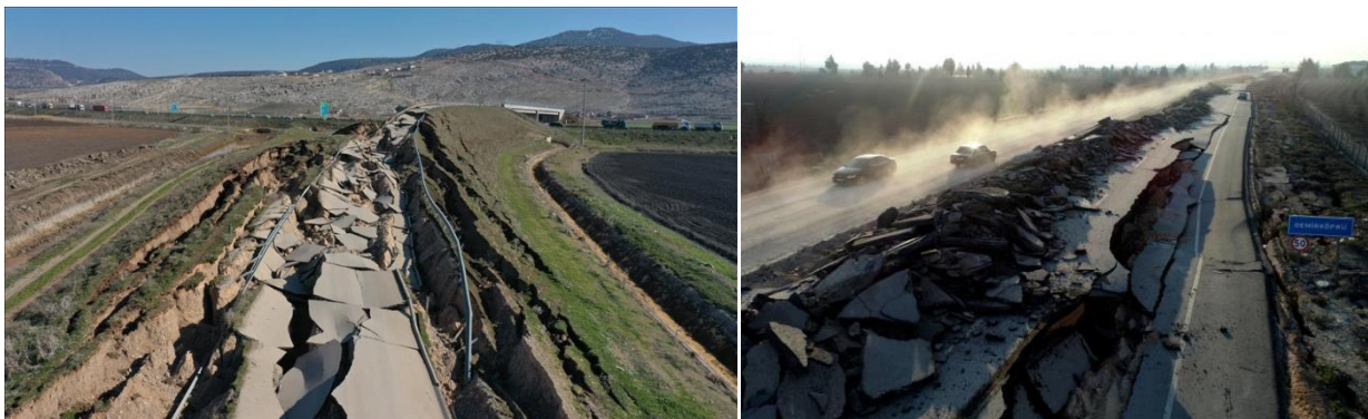
Figure 1. Road damages caused by the earthquake in Kahramanmaraş and Hatay.[URL1; URL 2]
