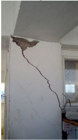
Figure 12. Short column damage in our study
